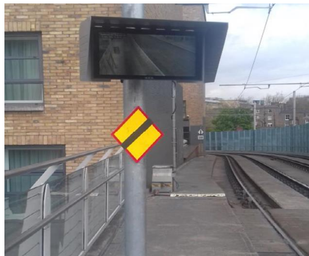
Figure 9 – Charlemont CCTV Monitor
