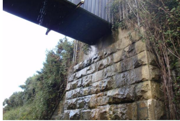
Photograph 4 – Water pouring down the parapet of the footbridge
