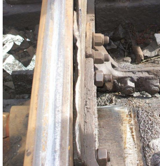
Photo 2 – Damaged switch rail
