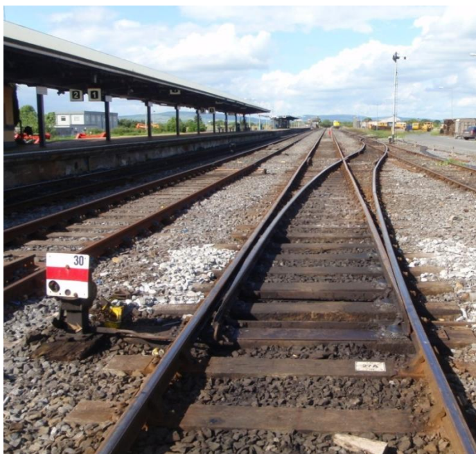
Photograph 1 – Points at Limerick Junction
