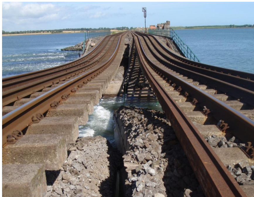
Photograph 3 – Malahide Viaduct Collapse
